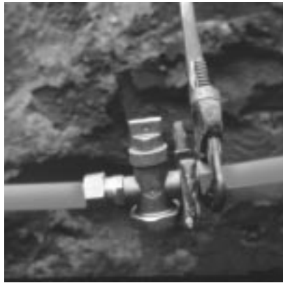
Fig. 4.3: MUNICIPEX installed with regular corporation brass
